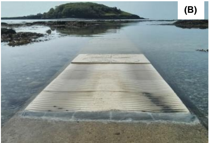
Outfall pipe on Hannafore beach in West Looe, Cornwall
